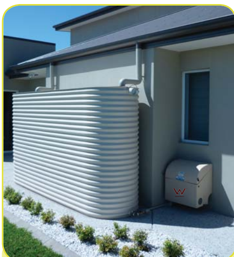
EXAMPLE OF WATERMARKED ACTION SWITCH BOX INSTALLED
